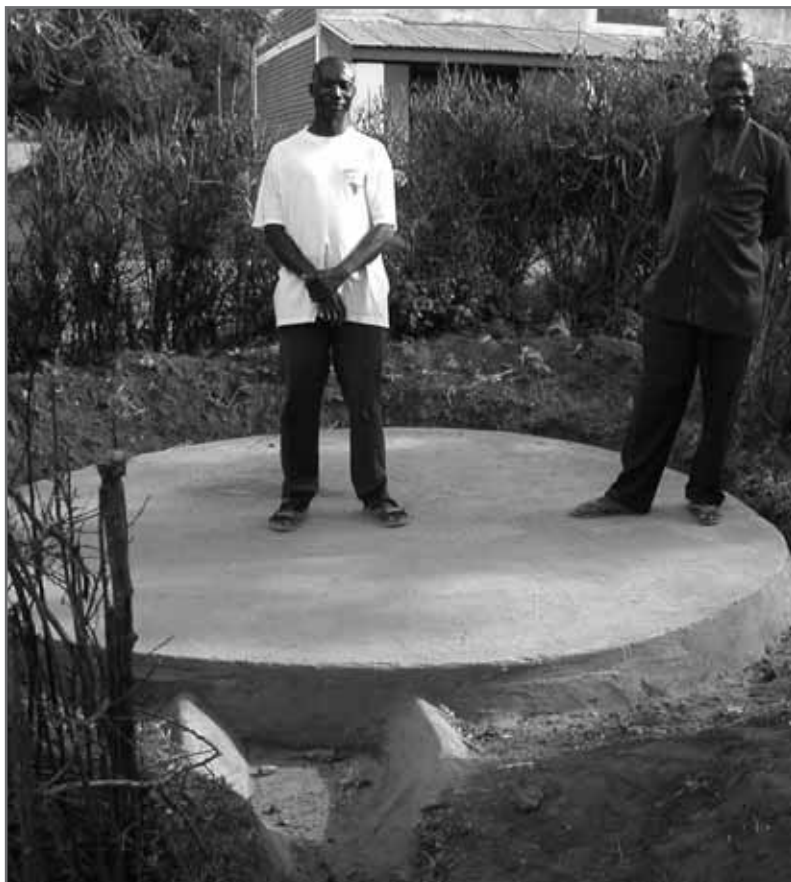
Community members in Migori stand on the foundation they have just built for a new water tank for their local dispensary.
