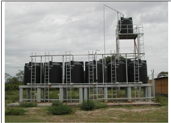
Water Facility at Songosongo Dispensary: This water facility receives clean water (sea water processed and treated at Songosongo gas plant to be clean for human use). The water is then distributed to the 5 water points/kiosks around the village from this facility.
