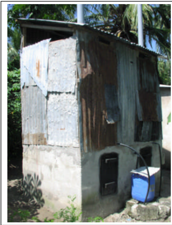
Photo 4: EcoSan toilet with Corrugated iron sheets
