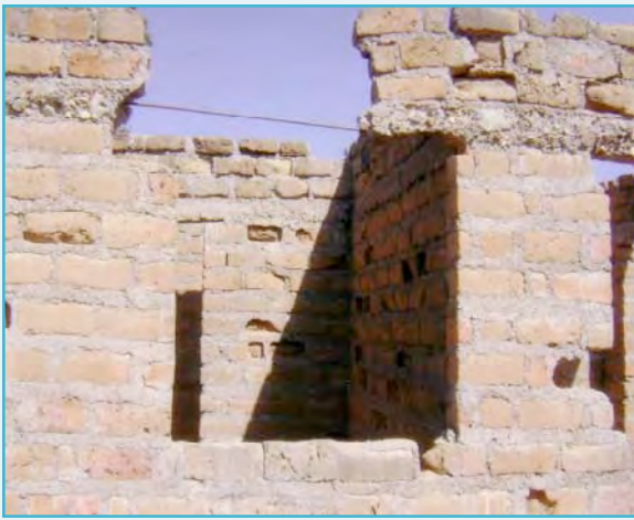
A nearly collapsing teachers' house at Fogofogo Primary School in Nyamikoma, Magu.
